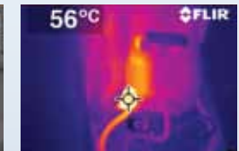
What a thermal imaging camera sees.
