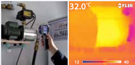
Thermal imaging allows you to quickly identify electrical and mechanical problems.
