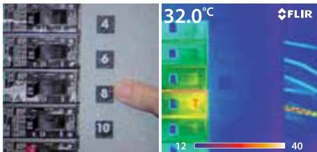
Bad connections are invisible to the naked eye but are clearly seen on the thermal image.
